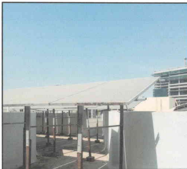
Photograph of Roof Top Solar PV Plant:
