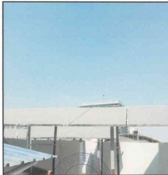
Photograph of Roof Top Solar PV Plant:
